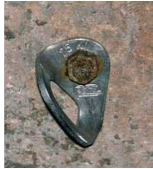
Rusting mild steel expansion bolt. All bolts and hangers should be stainless steel.
