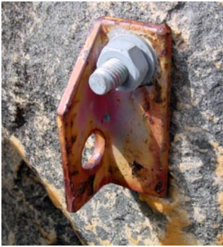
Homemade hanger on mild steel bolt. All bolts and hangers should be stainless steel and hangers should conform with EN-959.
