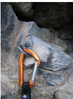
Example of a Sub-Standard Anchor. While the anchor assembly complies to EN 959, the fractured rock becomes the weak point.
