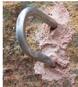
Worn and poorly placed U-bolt. Anchors with any visible signs of wear should be immediately replaced.
